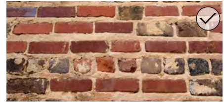
Re-point mortar joints where there is evidence of deterioration.
