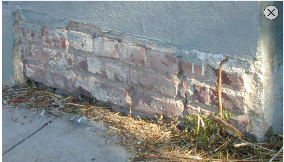
Do not allow an original foundation to fall into disrepair.
