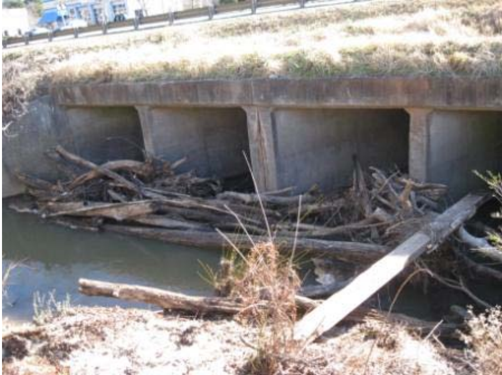
Figure 5 - View of obstructed box culvert at Alpharetta Highway.
