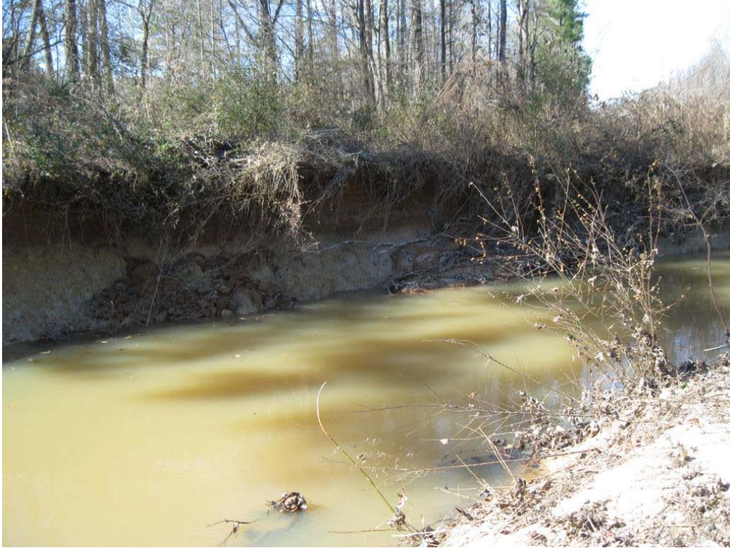
Figure 1 -View of streambank scour upstream of Upper Hembree Road.
