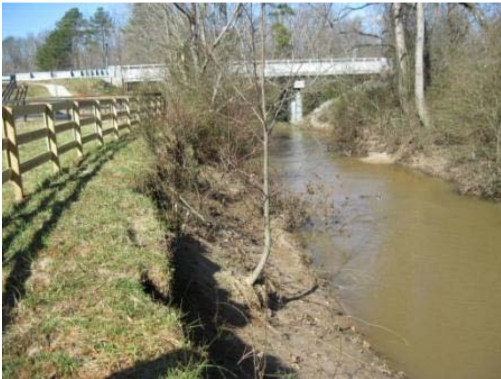
Figure 2 - View of upper bank failure south of Upper Hembree Road near horse farm.
