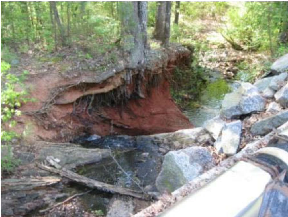
Figure 4 - View of erosion on tributary near Oak Chase.
