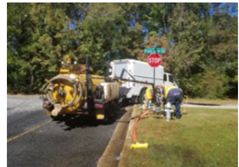
Photo of Crew Exercising a Valve
