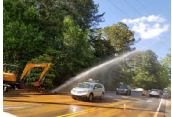
Photo of a Water Main Leak
