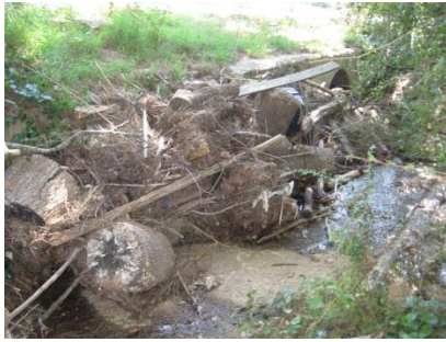
Photograph 1: Worthington Hills Drive culverts blocked by debris.
